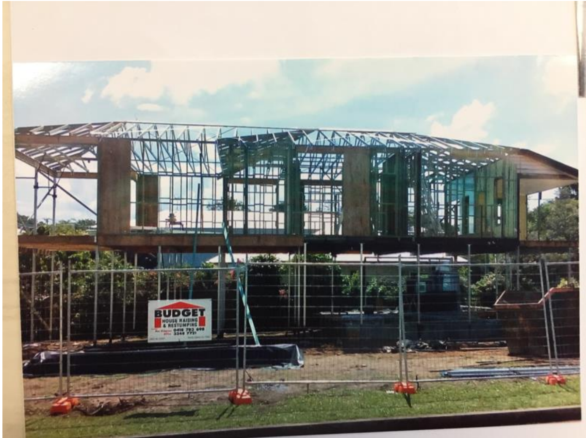
View from Albemarle Street during renovation. Note: the original house is roughly the right half of the structure and has been lifted moved westwards and rotated 90° to face north towards Soden Street.
